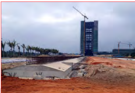
The tracks from the vertical assembly building to the launch pads under construction. The picture shows that the bed for one of two tracks has been almost completed. The vertical assembly building and another track are visible in the background at the left of the picture. (credit Chinese internet)
