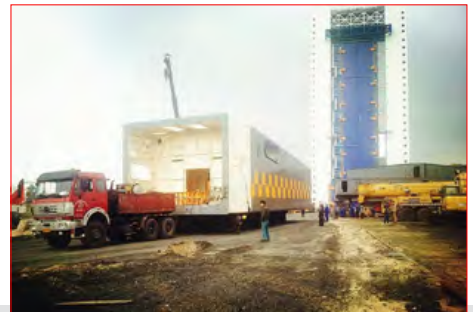
One of the umbilical towers still on the ground. Once installed on the launch platform, they will provide support of fueling, gas, air conditioning and power supply to the launcher. The VAB and the launch platform are seen in the background. (credit: Guangzhou Transportation Co. Ltd.)
