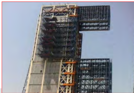
Full view of the CZ-5 launch tower, taken in early 2014. The tower had almost been completed when the photo was taken. Note, that there is no crane at its top, which is the first time for a Chinese launch tower. (credit: Chinese internet)
