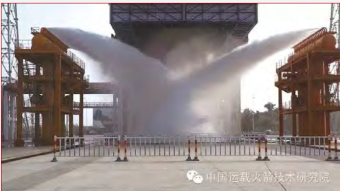
The level 2 water pouring testing at the CZ-7 launch pad. (credit: CALT/WeChat)
