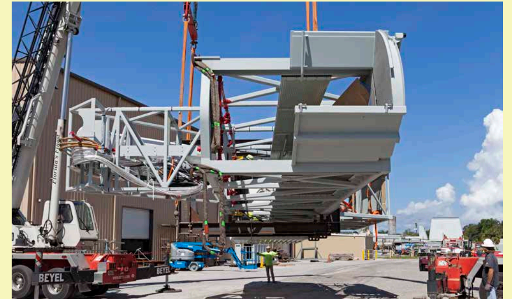
Two heavy-lift cranes are used to lower the Orion crew access arm onto a work stand in a storage location at Kennedy Space Center on Oct. 17, 2017. Photo credit: NASA/Kim Shiflett
