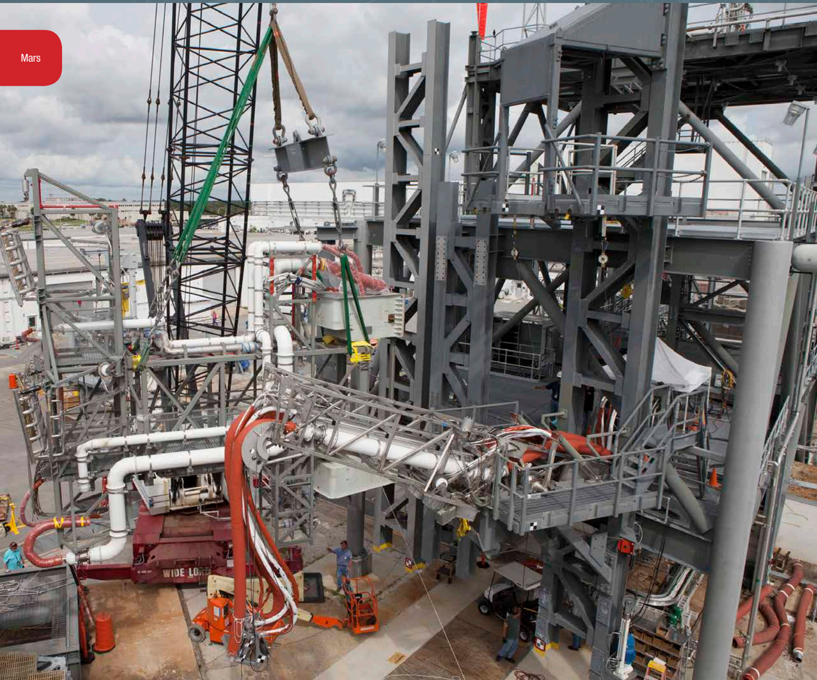
A view from above shows a heavy-lift crane attached to the Interim Cryogenic Propulsion Stage Umbilical at the Launch Equipment Test Facility, or LETF, at Kennedy Space Center. Photo credit: NASA/Glenn Benson
