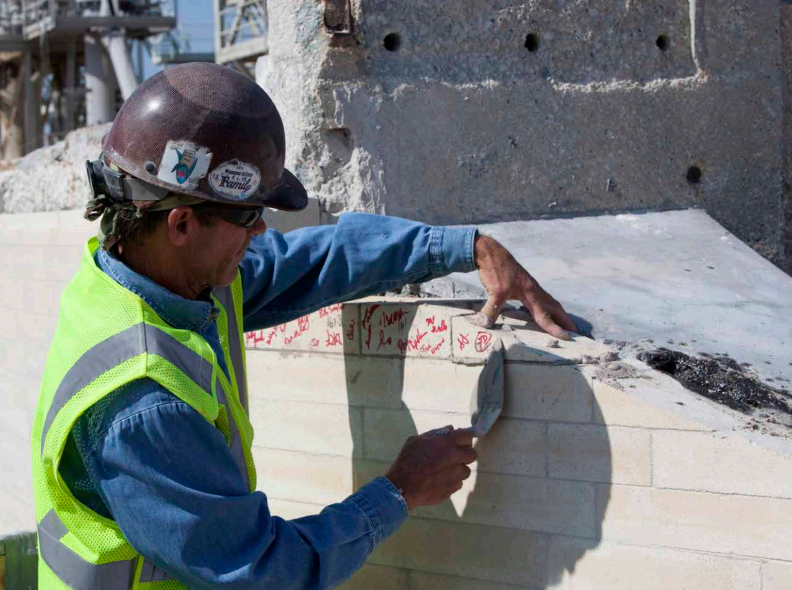
Jimmy Saylor, a mason with Reintjes Services, a subcontractor to JP Donovan, installs the final brick on the north side of the flame trench wall at Launch Complex 39B at Kennedy Space Center. Photo credit: NASA/Leif Heimbold
