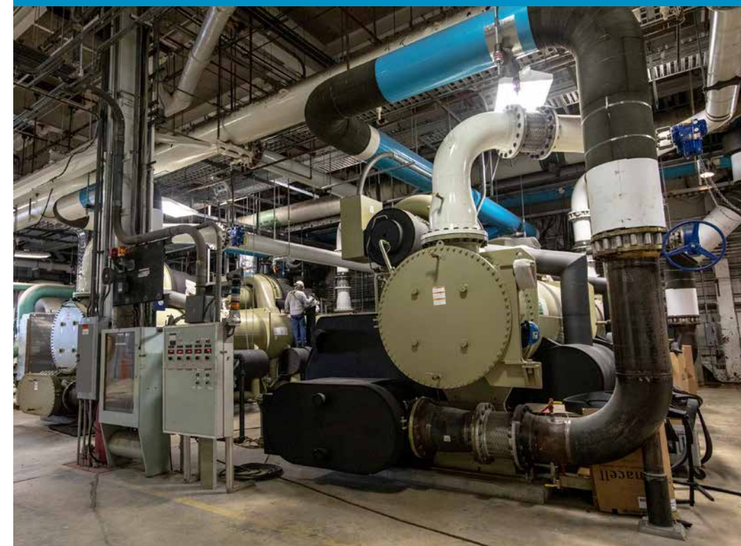
A view of the inside of the Utility Annex near the Vehicle Assembly Building at NASA's Kennedy Space Center on July 24, 2019. Photo credit: NASA/Kim Shiflett
