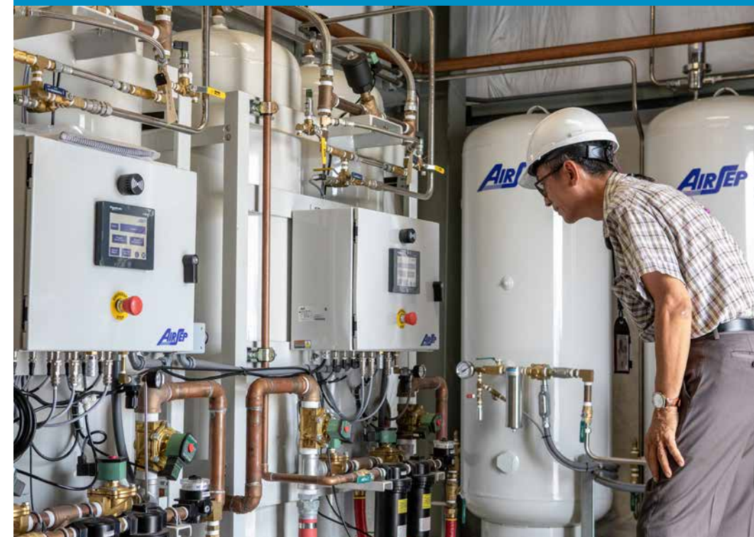
A photograph taken July 24, 2019, shows new air tanks, piping and control panels were installed in the Utility Annex near the Vehicle Assembly (VAB) Building at NASA's Kennedy Space Center. The Utility Annex, which provides 8,000 gallons of chilled water per minute to the VAB and other facilities in the Launch Complex 39 area, is being upgraded and repaired. The facility also contains boilers necessary to provide hot water to the VAB. The center's Engineering Directorate is making the repairs and upgrades to the facility to prepare for the agency's Artemis missions to the Moon and on to Mars. Photo credit: NASA/Kim Shiflett
